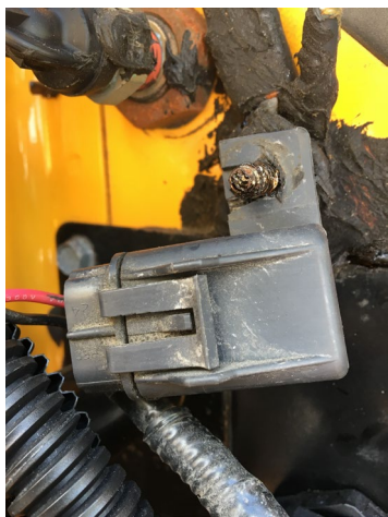
Fuse Holder and 10A Fuse. Mount the fuse holder against the bulk in a location that is accessible for service
